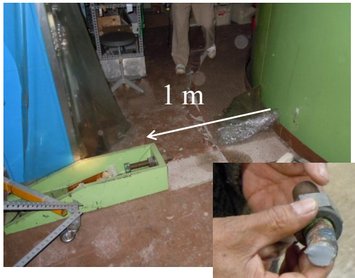
Figure 3: Broken shock prevention device for the accelerator tank at the 7th floor. Anchor bolts of 1 inch in diameter for the shock prevention device were severed by the shock of the earthquake.
